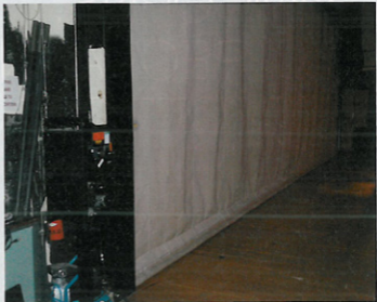
Firewall? Special effects seem to be a part of any performance these days. Some of them involve a risk of fire. The image above shows how a fire curtain lowered in proscenium opening can isolate any stage accident from the audience.
